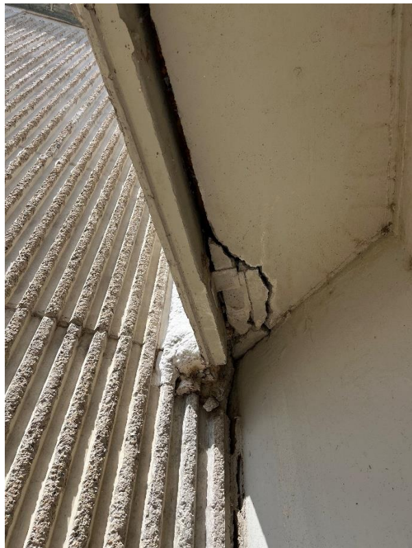
Figure 11-50: Seismic Damage at TF Digesters
