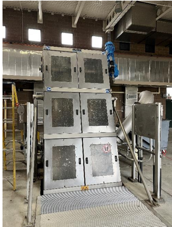
Figure 11-8: AS Headworks Influent Screen
