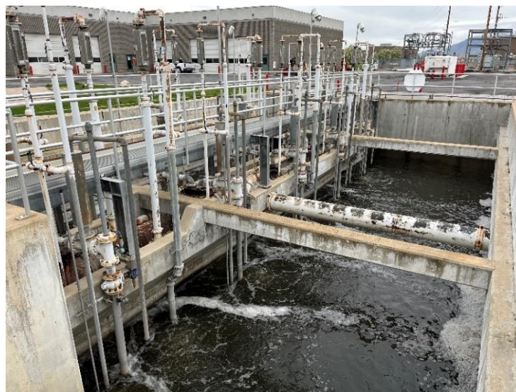
Figure 11-28: TF Headworks Aerated Grit Basin
