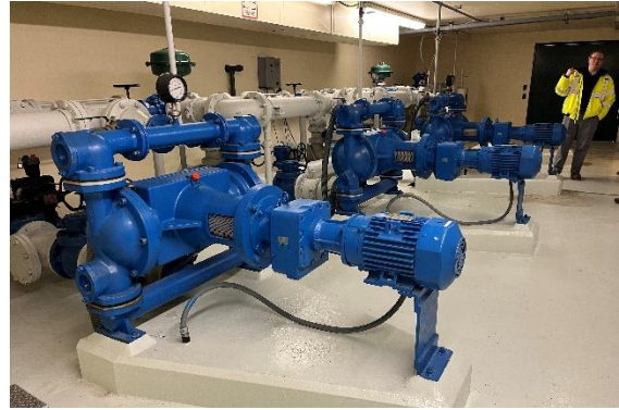
Figure 11-32 TF Primary Sludge Pump Station
