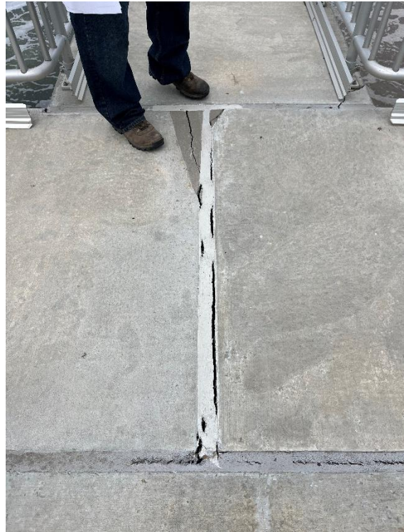
Figure 11-53: Cracking Noted at AS Aeration Basins
