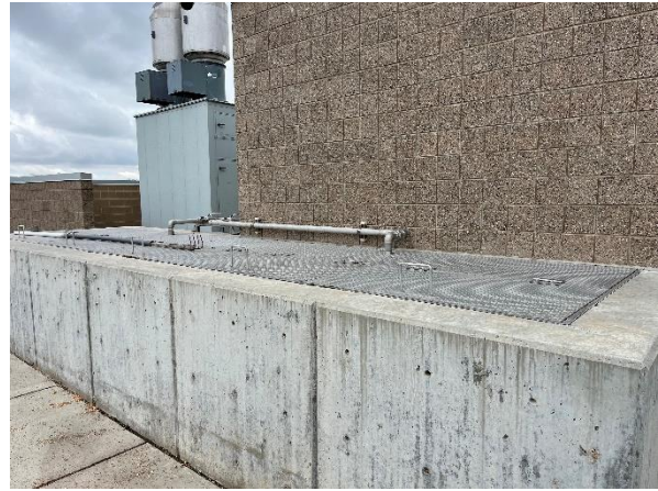
Figure 11-55: AS RAS/WAS Pump Station Scum Box
