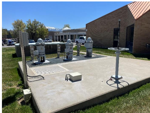
Figure 11-36: Humus Return Pump Station
