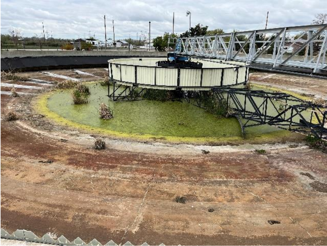
Figure 11-35: TF Final Clarifier No. 3
