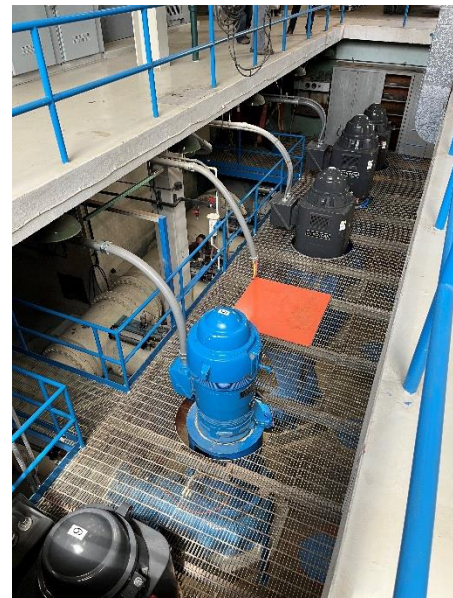
Figure 11-29: TF Influent Pump Station
