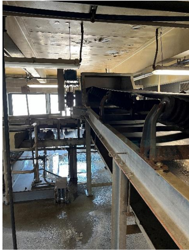
Figure 11-57: Dewatering Building Second Floor Ceiling
