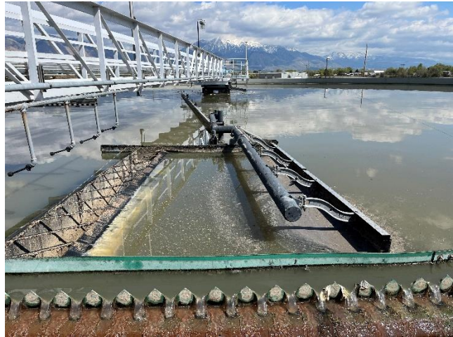
Figure 11-52: AS Primary Clarifier Scum Beach
