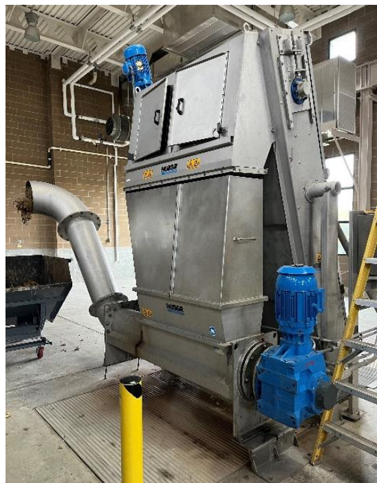
Figure 11-9: AS Headworks Screen and Compactor
