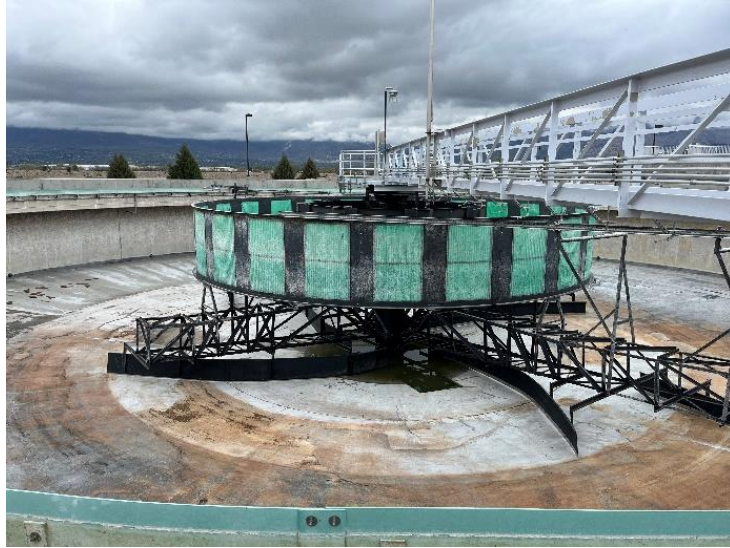
Figure 11-15: Secondary Clarifier Mechanism
