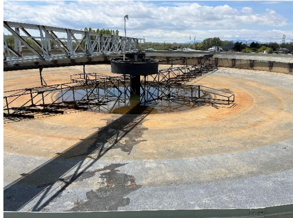
Figure 11-31: TF Primary Clarifier
