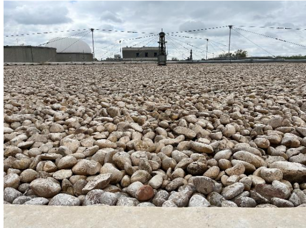
Figure 11-33: Existing Trickling Filters
