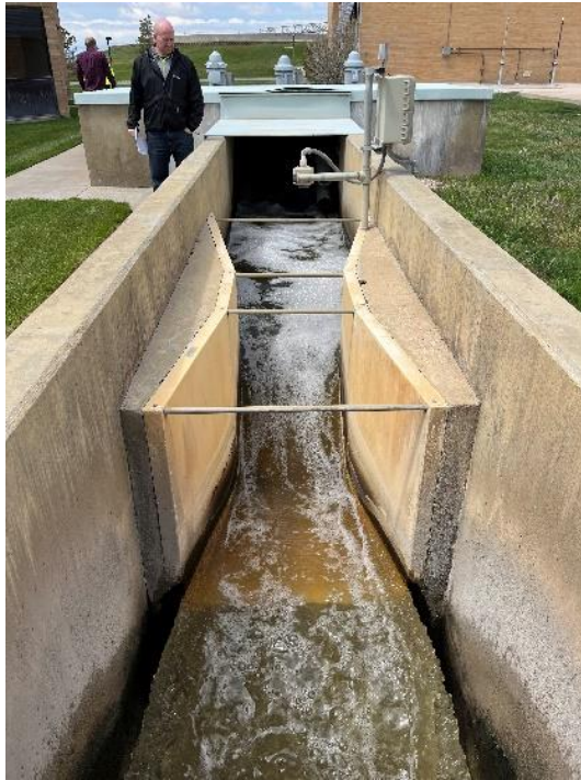
Figure 11-5: Humus Return Parshall Flume
