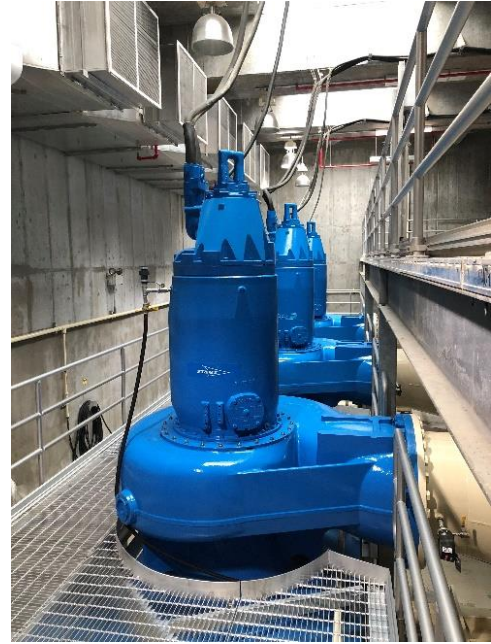
Figure 11-11: Inlet Pump Station
