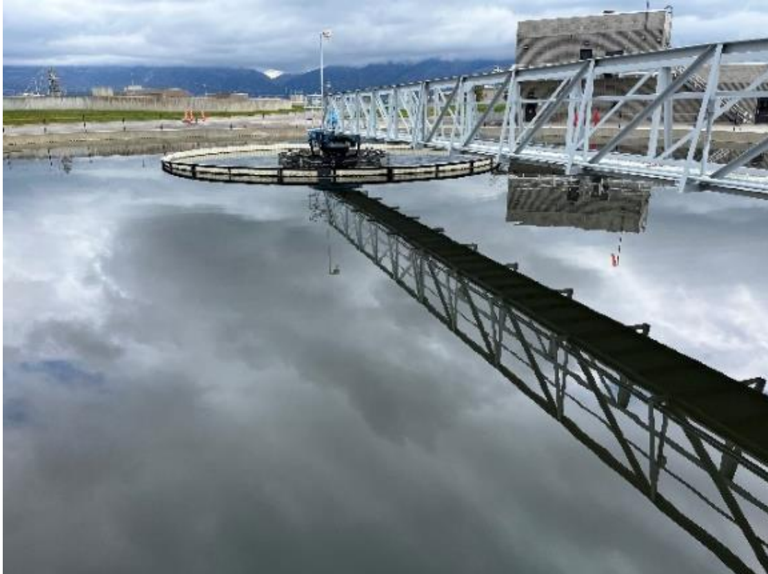
Figure 11-34: TF Final Clarifier No. 4
