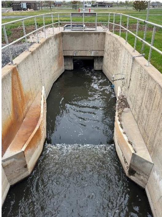
Figure 11-4: TF Headworks Parshall Flume
