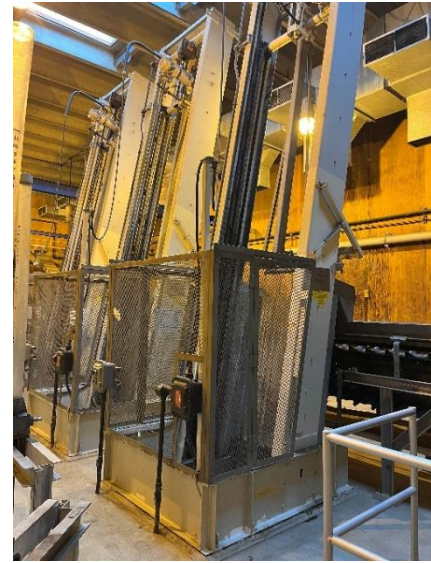
Figure 11-27: TF Headworks Screen
