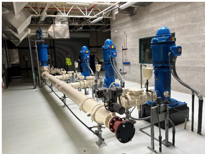
Figure 11-37: TF Utility Water Pump Station
